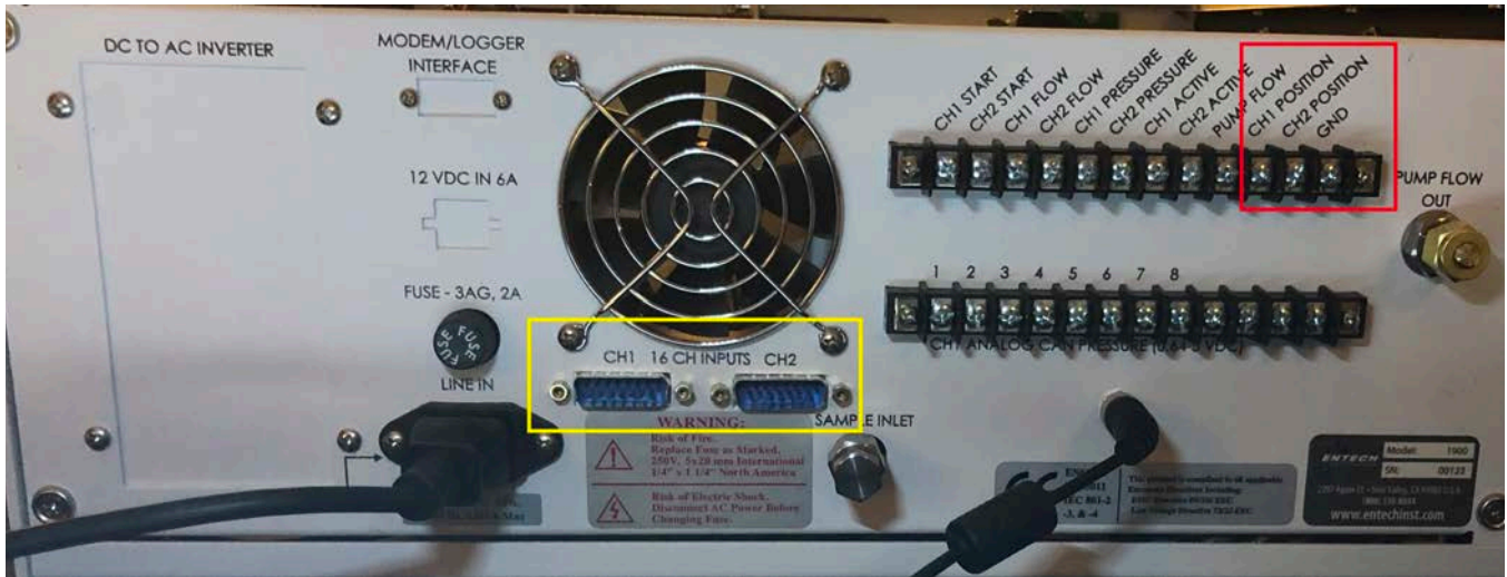
Figure 6.3.3. The red box shows the test points on the rear of the 1900 for the 1916 encoder voltage. The yellow box shows the connect points for the cable between the 1900 and the 1916.
